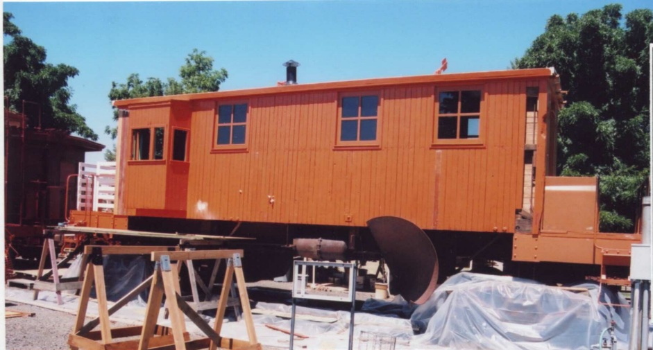
[LEFT] This is how our SP Flanger looked on 7/31/07. To the casual observer it looks very good, but not good enough for project coordinator Steve Bruff.
