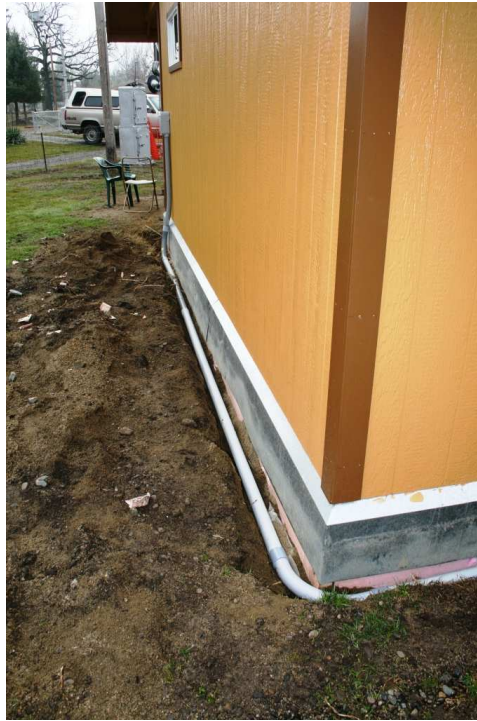
(LEFT) These two photos show the new electrical lines that will provide power from the SP Section Tool House to our new Mack Walch Archives building. While the digging along the Tool House was tough (far left), the digging along the new archives building was easier to do.
